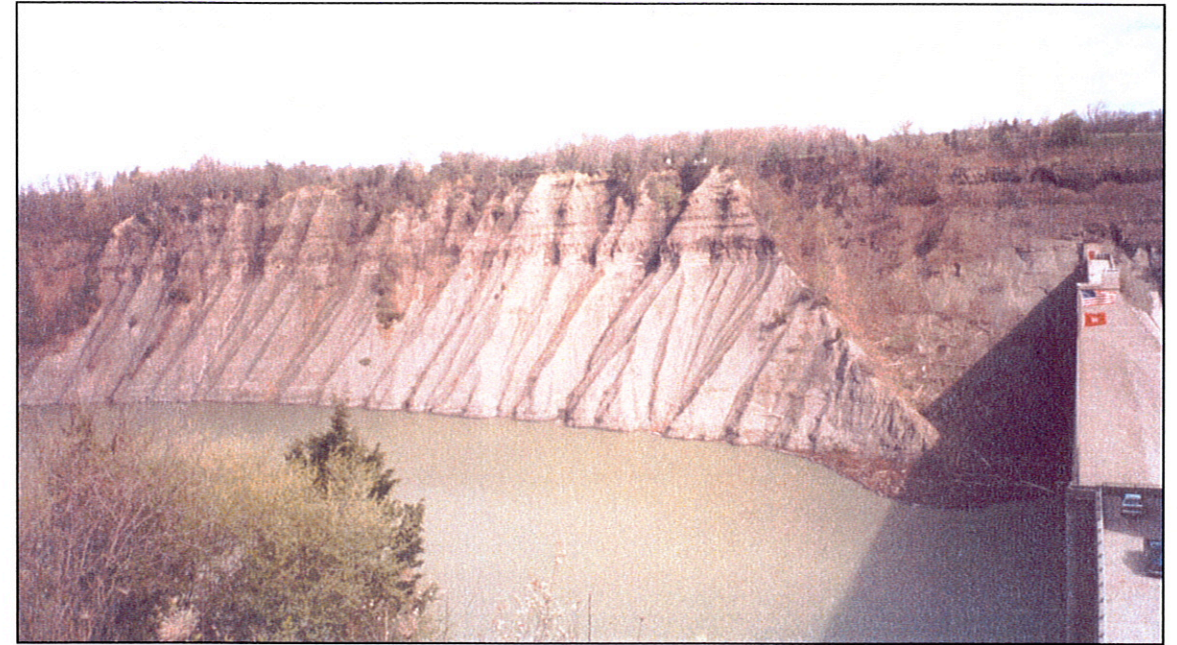
This is a picture of the Mount Morris Dam. Notice that the river caused some erosion.
