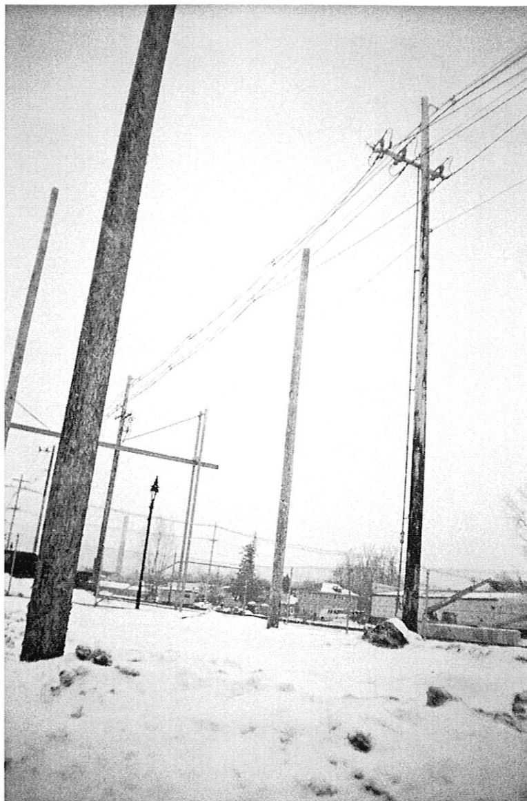
This is a switch pole. It was taken at Fairport Electric on Monday, February 12, 2007. It holds electricity wires.
