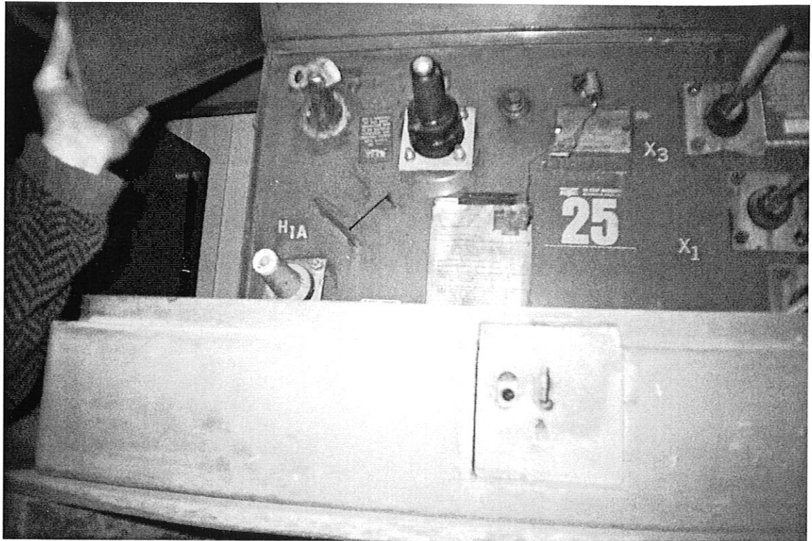
This is a transformer. It was taken on Monday at Fairport Electric. My transformer goes to another transformer.
