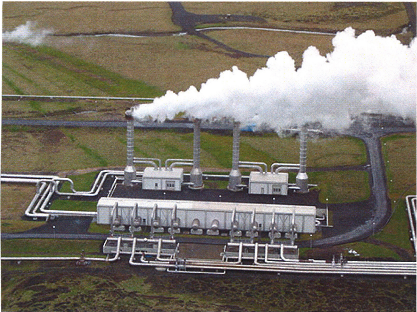
Geothermal power plants tap into the naturally occurring heat trapped inside the Earth.
